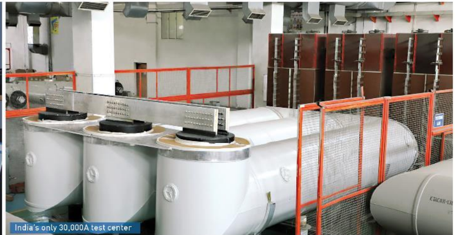
India's only 30,000A test center
