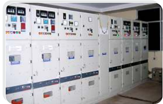
11kV Indoor VCB Panel
