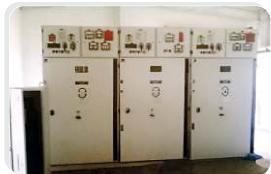
33kV Indoor VCB Panel
