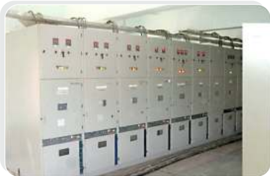
22kV Indoor VCB Panel
