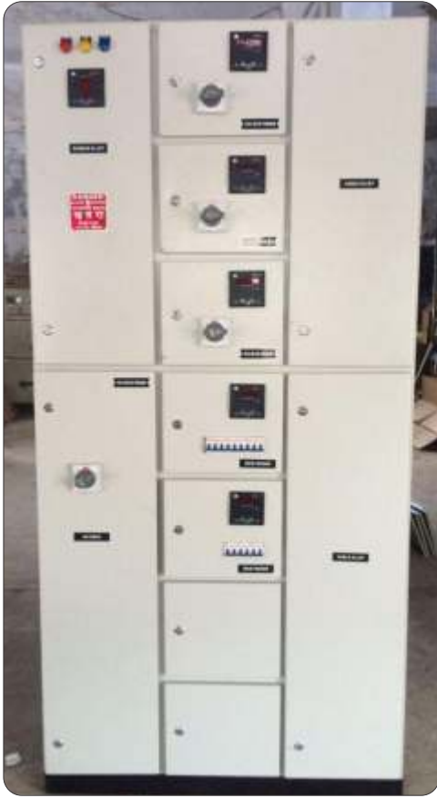
CSM Meter fixed on the Panel
