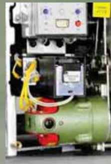
Motor / Remote connection
