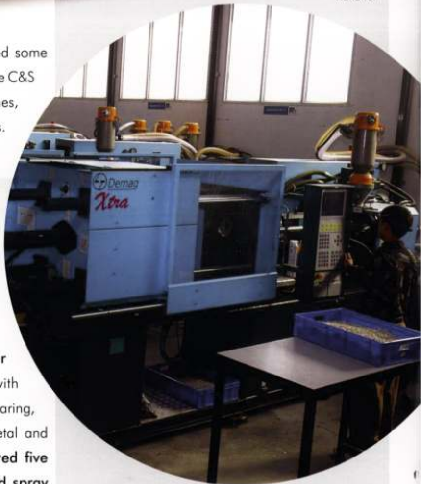
CNC injection moulding machines (Demag) Haridwar
